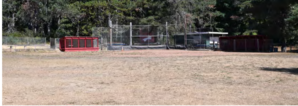
Baseball field does not have irrigation. The grass area needs regrading and reseeding. Backstop, bases, dugout and scorekeeper's booth are worn. Estimated cost.....$125,000-160,000 » Baseball field upgrades, ADA improvements.
