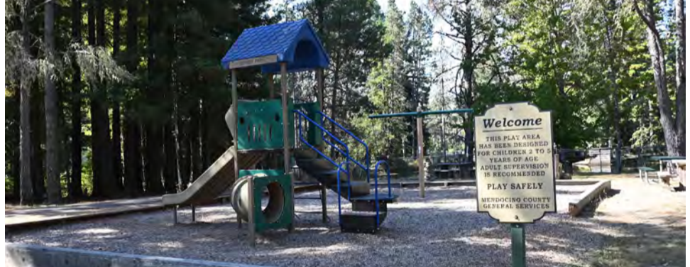
Protective surfacing needs replenishing, wooded edge is failing. There is no safety fencing around the play area. Estimated cost..... $50,000-80,000 » 2-5 Play area upgrades, 5-12 upgrades, ADA improvements.
