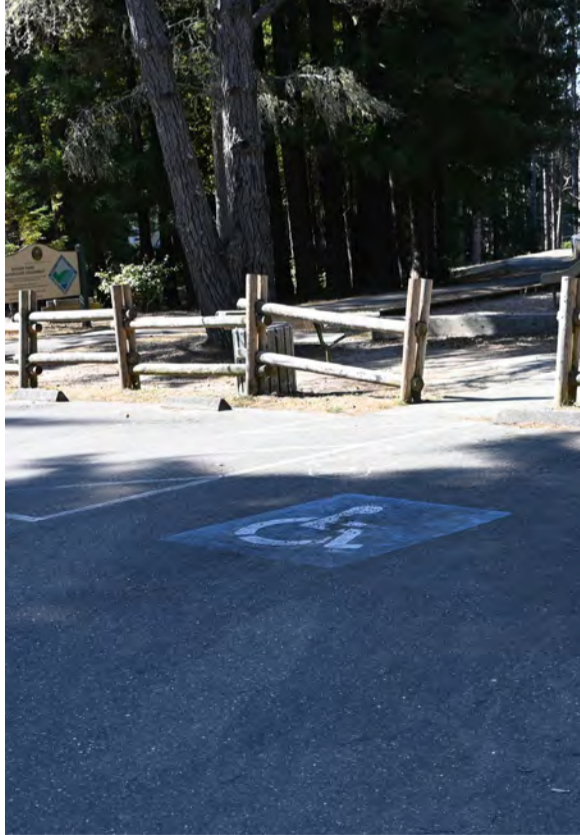
The striping in the parking lot is worn and hard to see. Est. cost..... $100,000-140,000 » Parking lot sealing and restriping.
