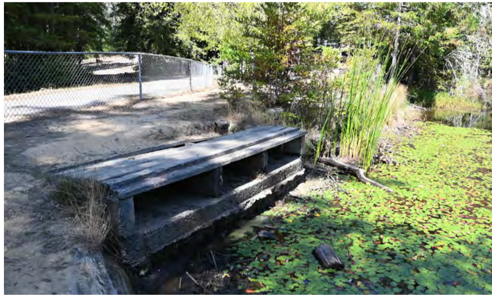
Spillway is damaged and cannot support pathway and pedestrian traffic that goes around pond. Estimated cost.....$60,000-90,000 » Spillway repair., structural considerations (concrete), repave.
