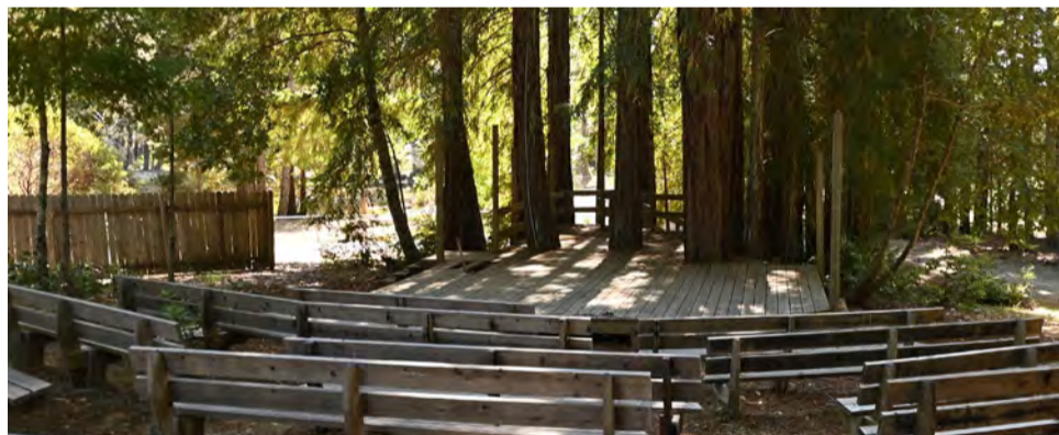
The stage of the amphitheater is damaged and there is no ADA access to it. Some seats need repair. Estimated cost.....$25,000-35,000 » Demolition of damaged structures.
