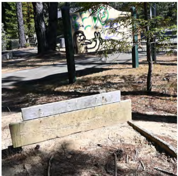
Horseshoe pit is in disrepair. Est. cost.....$8,000-10,000 » Relocate, construct the horseshoe pit.
