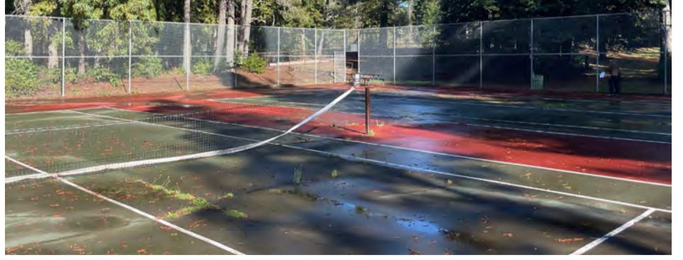
Tennis court is damaged and needs repair. Nets are missing, fencing is damaged. ADA improvements. Estimated cost..... $100,000-125,000 » Demolition of court, repave, striping, fencing, pickleball, ramp.
