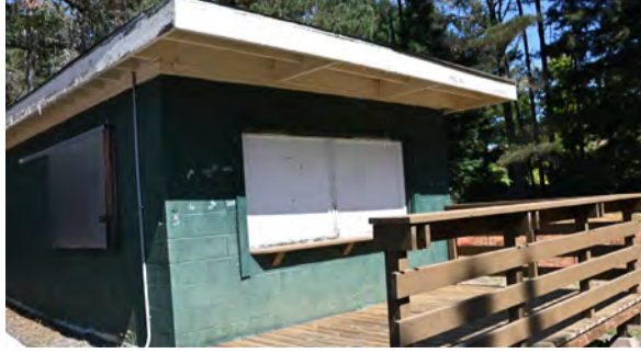
Concession stand needs new roofing and ADA access. Est. cost.....$50,000-80,000 » Concession stand repairs and ADA .
