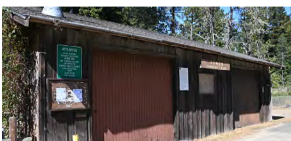
Community building needs many upgrades. Demolition was determined to be more cost effective. Est. cost $30,000-55,000 » Demolition of the building
